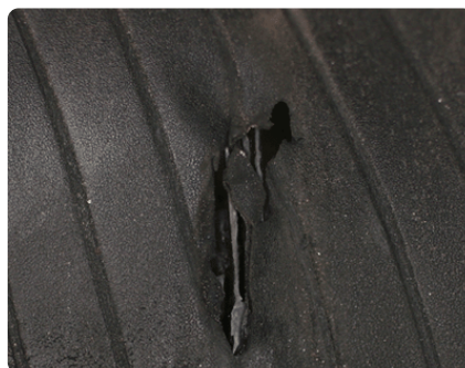
1 or 2 Pictures of INSIDE OPPOSITE OF THE DAMAGED AREA
